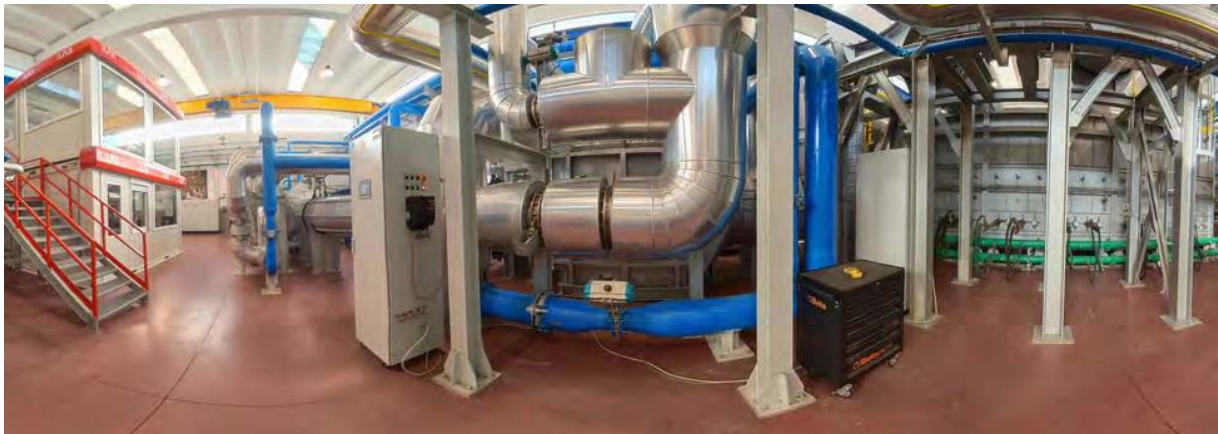
Figure 3. Tenova T-Lab panoramic picture showing the control room for enhanced automation and digital applications (left), the waste gases and heat recovery system (middle) and one of the test furnaces (right).
